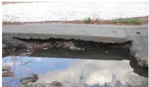
Old Spillway weir before repair.
