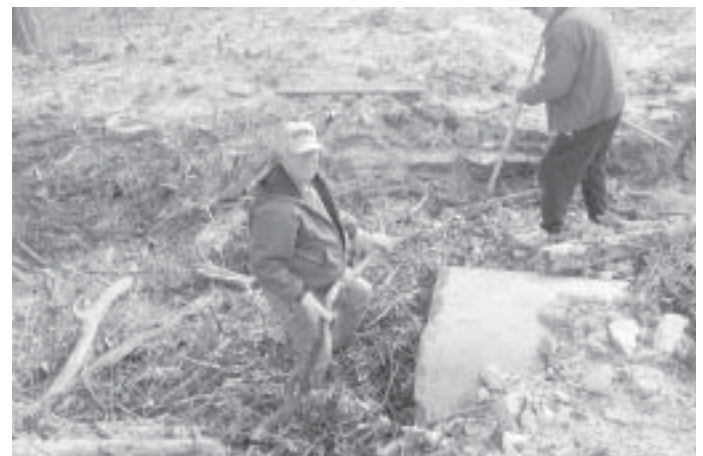
Volunteer Day, March 18. Ken Jost and Lou Harting clean debris from the culvert pipe at the southside bridge.
