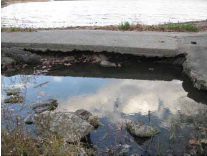
The old weir (viewed from the spillway channel) was severely undercut from many years of erosion.
