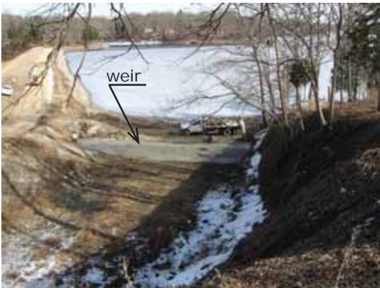
Workers finish construction of the new spillway weir. See page 7. More photos at
