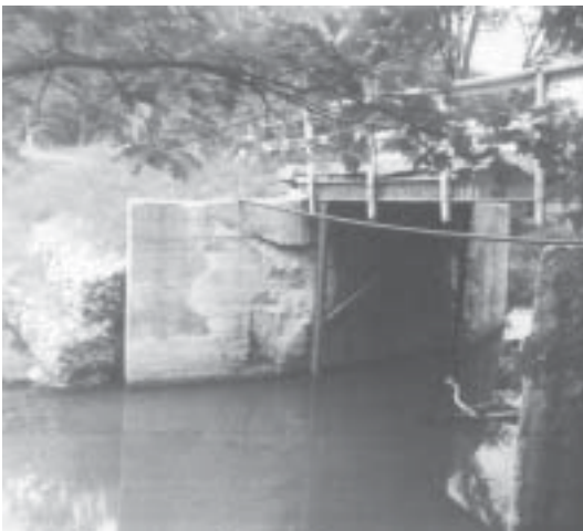
Photo of southside bridge from 1993. CRD Campbell Engineering comments: View of the north abutment. Note the poor condition of the concrete-much has spalled away and very little reinforcement is evident. Bridge superstructure is supported on the steel piles. Viewed looking northeast.
