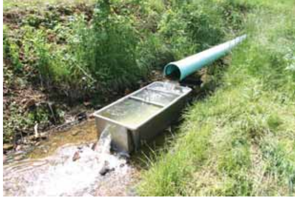
Weir box, constructed by Mike Leiweke, capturing leak flow at 300 gpm, before repair
