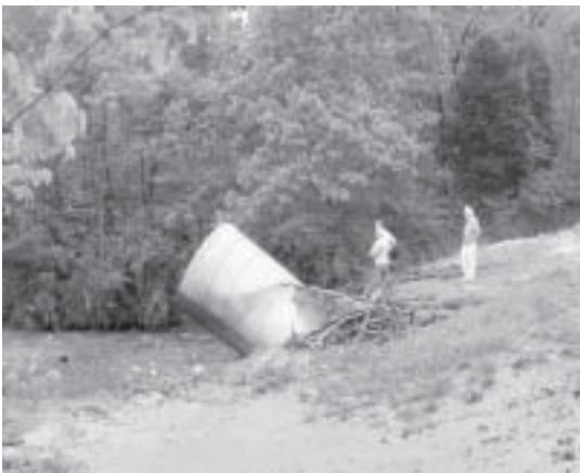
The great flood of May 2003 upended the culvert pipe that passes under South Lakeshore Dr. Viewing the pipe are Butch Hopfer, Dale Farwig, and Lou Harting.
