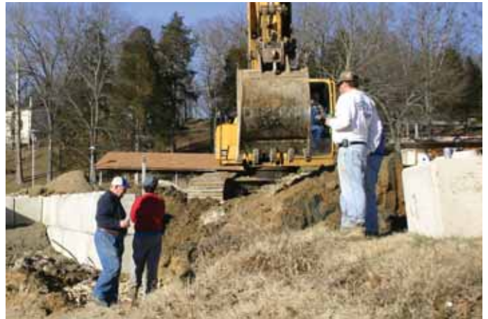
Henry, at left, helping with the construction of the lakefront seawall February 2006.
