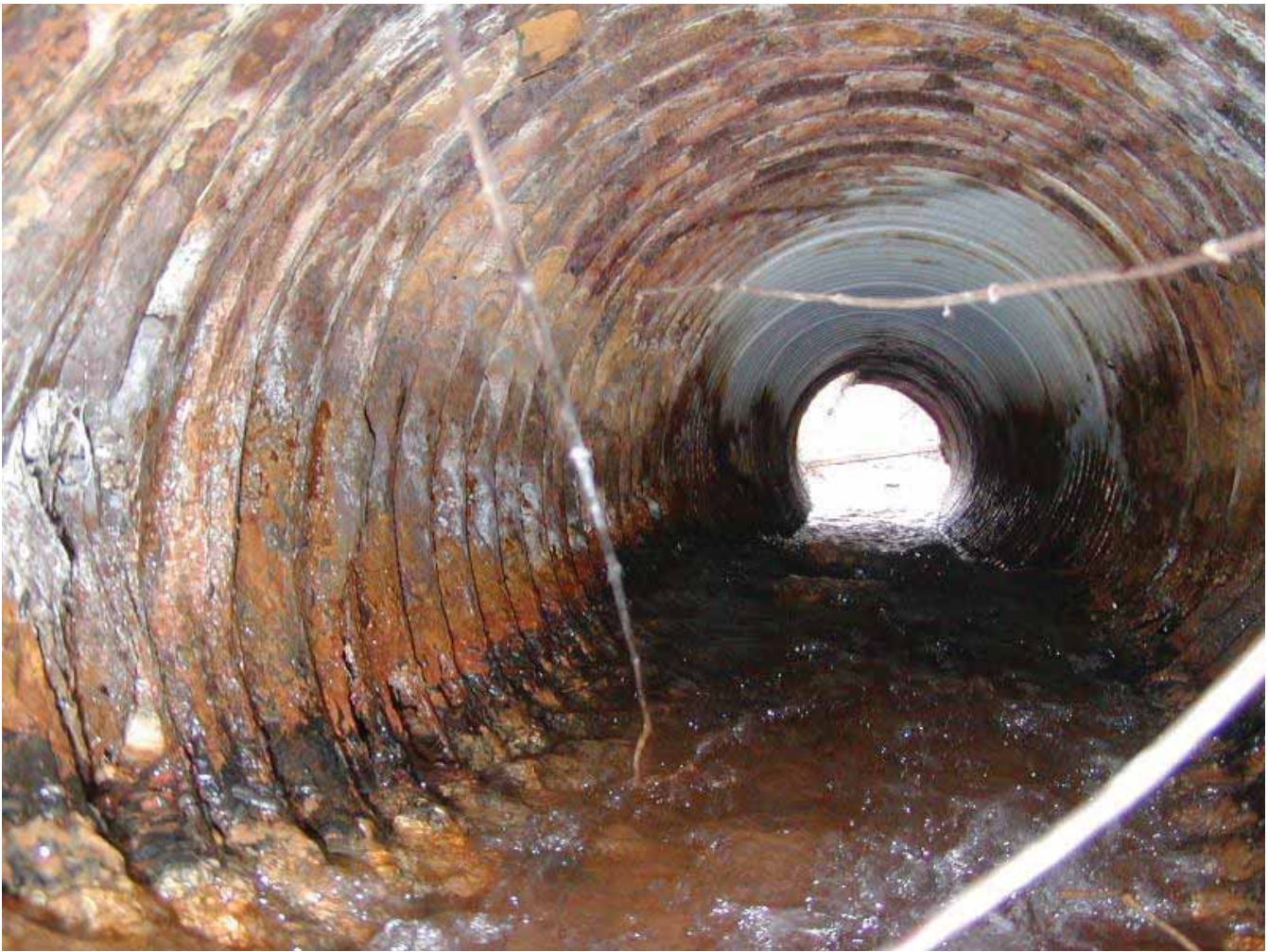
Above: View thru 24" x 20' drainage pipe, from leak pool.
