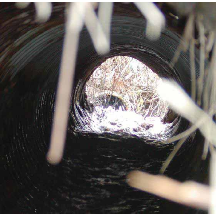
Left: View thru 24" drainage pipe, toward the leak pool. Leak outlet pipe is at center of photo.
