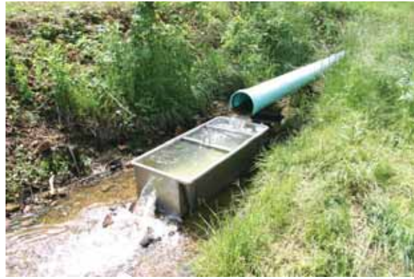
Weir box, constructed by Mike Leiweke, capturing leak flow at 300 gpm, before repair
