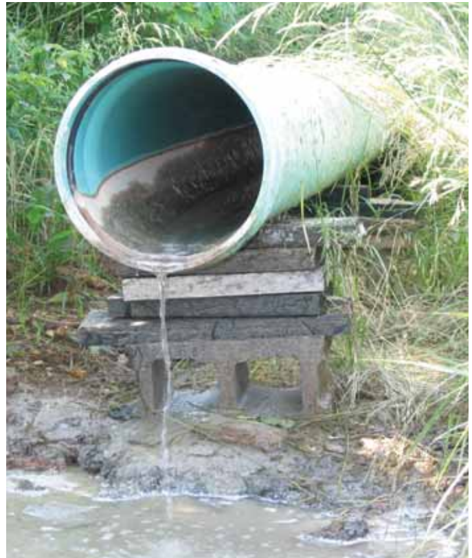
Water flow from leak collector, 0.6 gal/min, June 2008.
