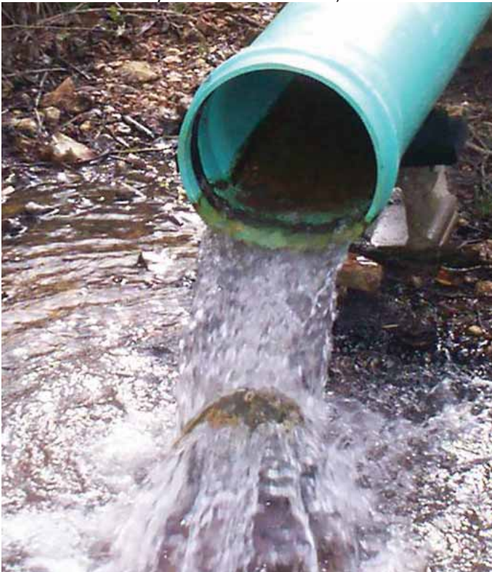
Water flow from leak collector, 300 gal/min, January 2008.
