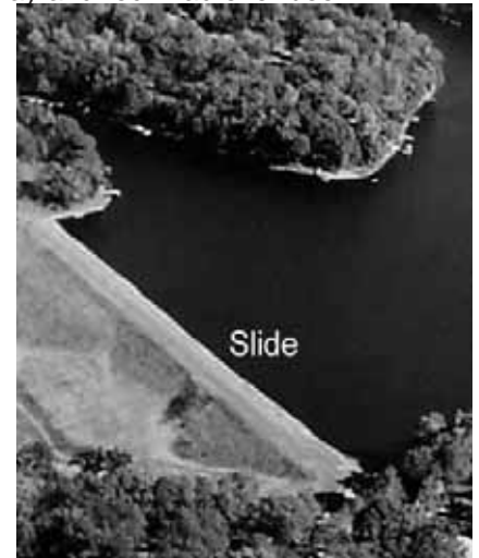
Figure 1. Slide on back of dam
